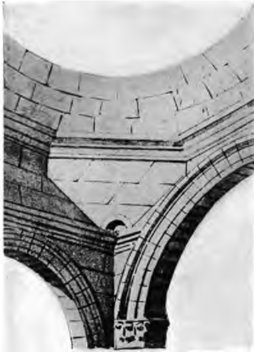
ILL. 75. — Smoothed Squinch of Arch at Latakia. (From Rivoira, by Special Permission)
